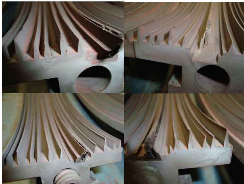
Figure 4 – Retractable Brush Seals after 7 Years of Operation
